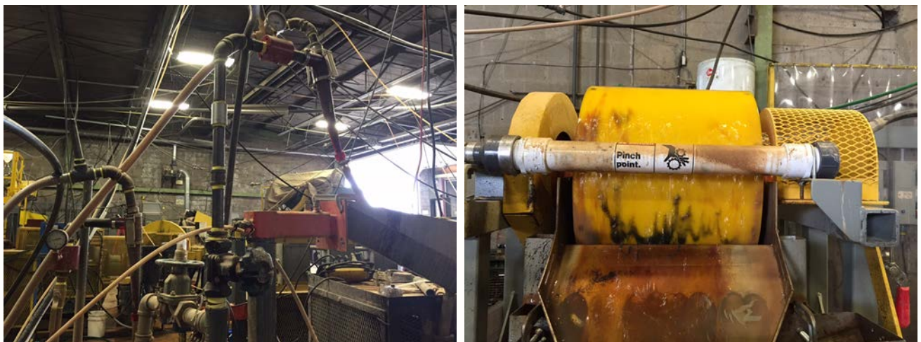
Figure 3: Integrated Pilot Plant Desliming and Magnetic Separation
