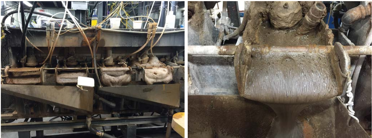
Figure 4: Integrated Pilot Plant Niobium Rougher and Cleaner Flotation Cells
